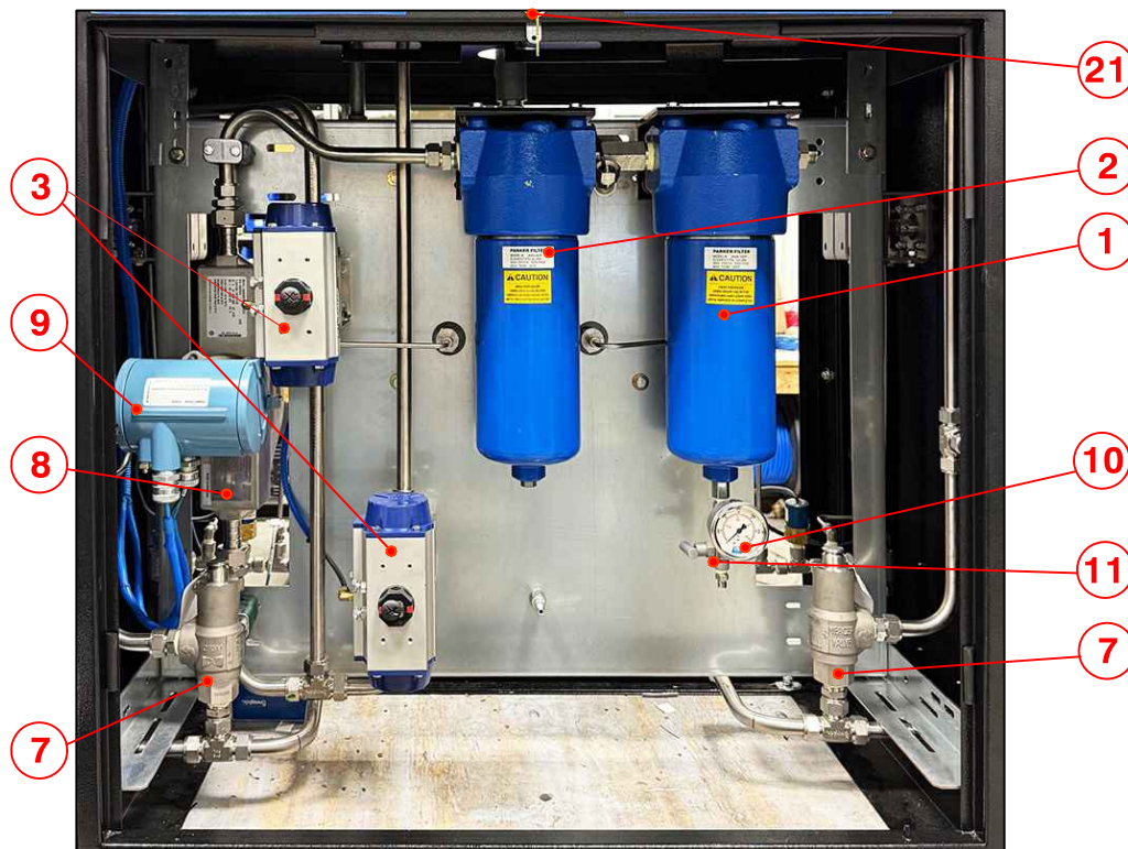
LOWER ENCLOSURE REAR
