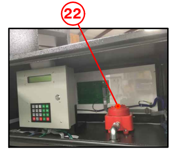
UPPER ENCLOSURE INTERIOR
